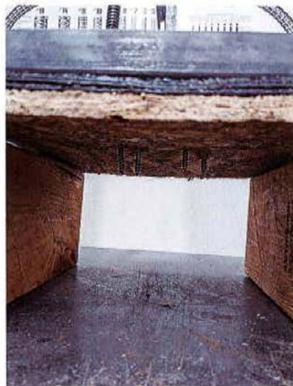
Figure 3c. Lag screw view of typical failure.
